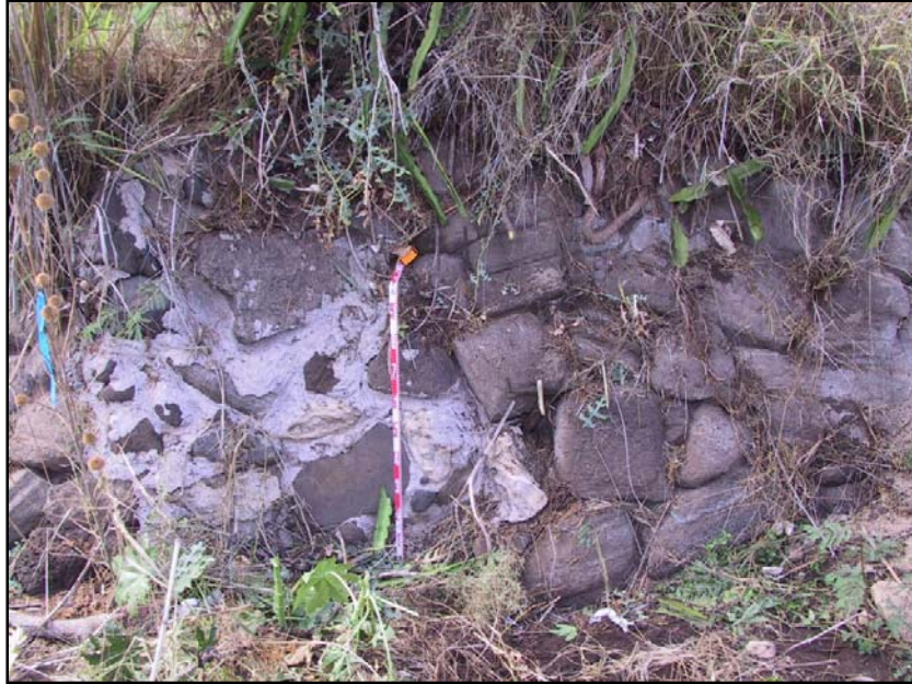
Figure 36. Photograph of the southern abutment of Feature B, SIHP # 50-80-12-9714, view south, showing crude basalt boulder and mortar construction
