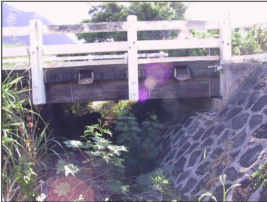
Figure 17. Photograph of SIHP # 50-80-07-6822, blue rock and mortar abutments with concrete reinforcement at corners; view north
