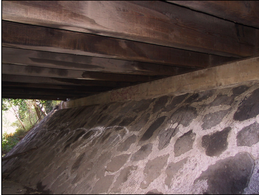
Figure 16. Photograph of SIHP # 50-80-07-6822, blue rock and mortar abutments, wooden beams and concrete end bent; view north
