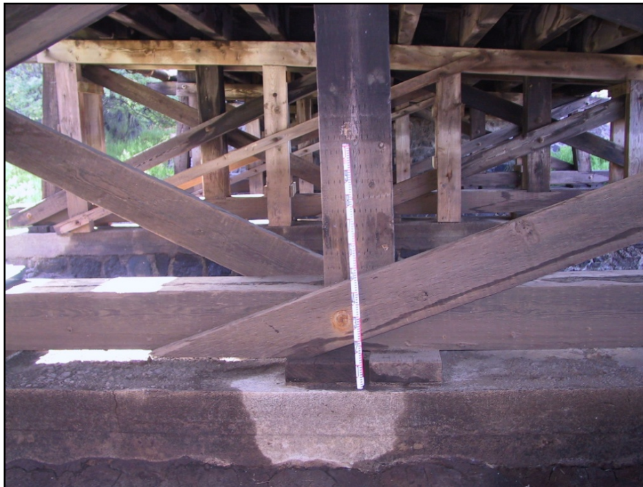
Figure 24. Photograph of SHIP # 50-80-07-6823 substructure, showing wooden columns, beams, planks, X-bracing, and the concrete and blue rock and mortar piers; view south
