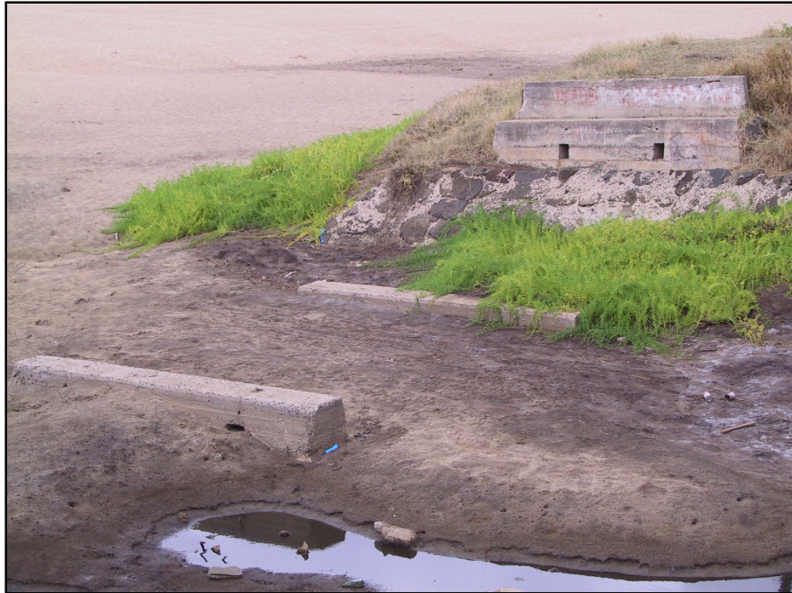
Figure 38. Photograph of the northern abutment and piers of Feature C, SIHP # 50-80-12-9714; view northwest
