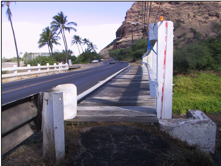
Figure 26. Photograph of SHIP # 50-80-07-6823, concrete corner reinforcement, wooden sidewalk and guardrail; view northwest
