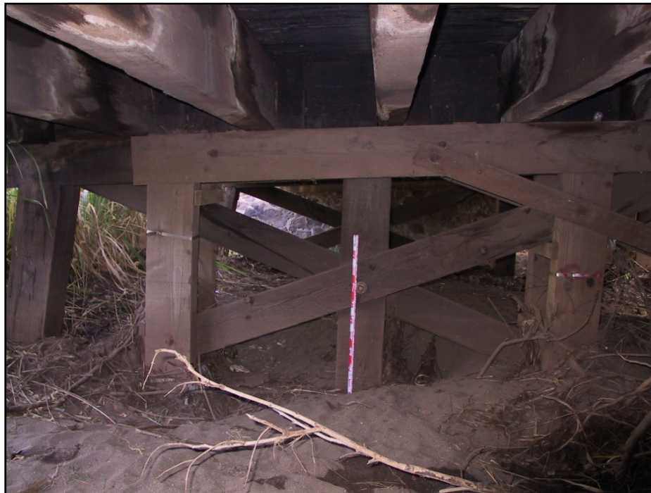
Figure 15. Photograph of SIHP # 50-80-07-6822, showing massive wooden beams, bents, and columns, and plank X-bracing, view to northwest/north
