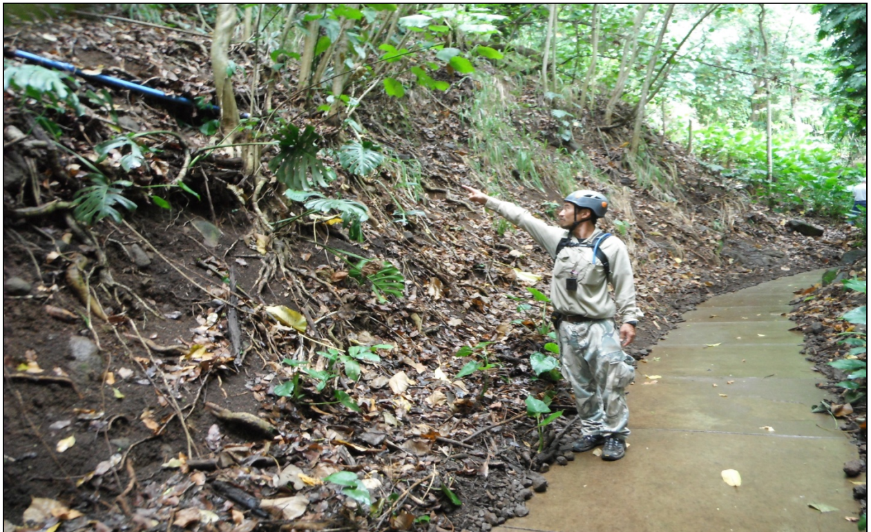
Rockfall Location 2 upslope from visitor's walkway; view to northeast.
