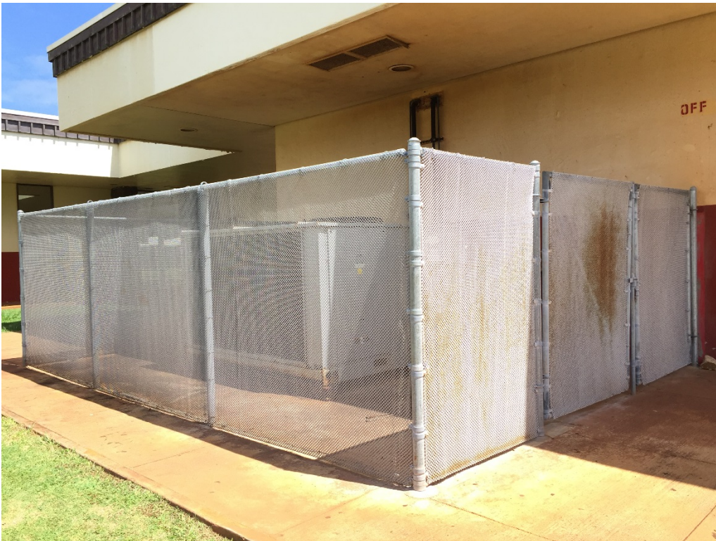
A/C chain link enclosure to be treated for rust and painted
