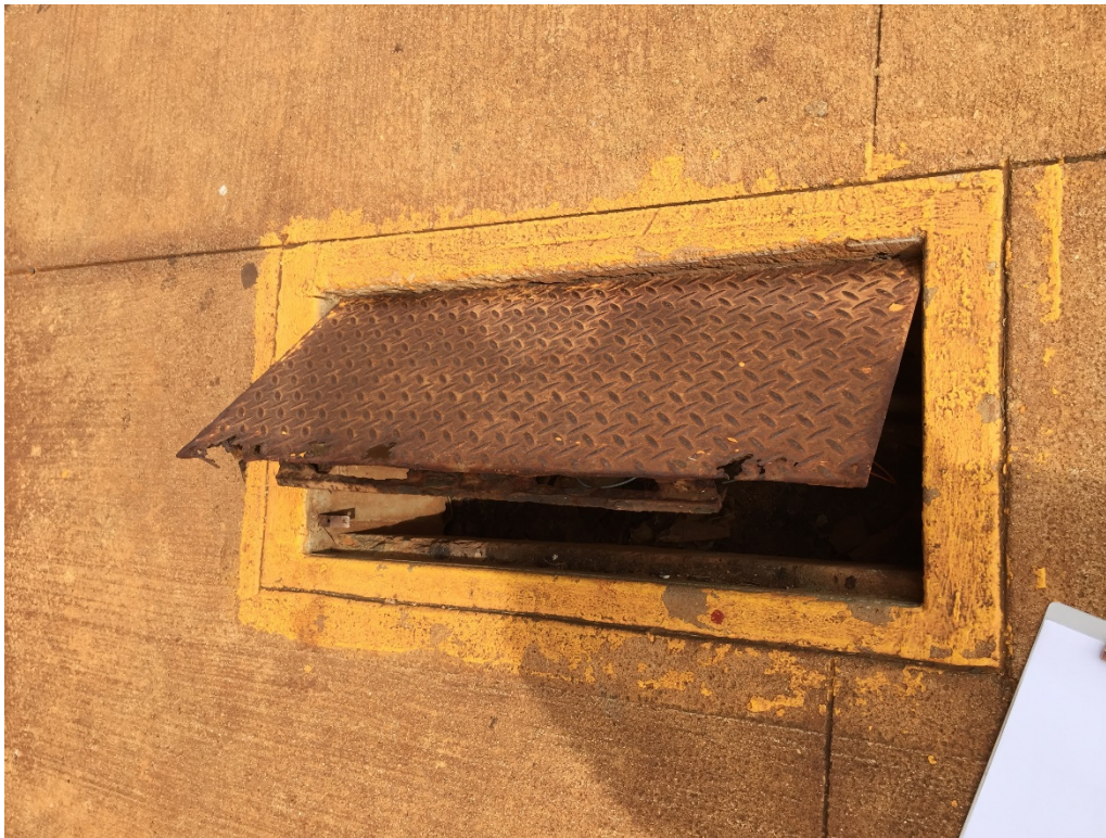
Steel diamond plate cover to be replaced
