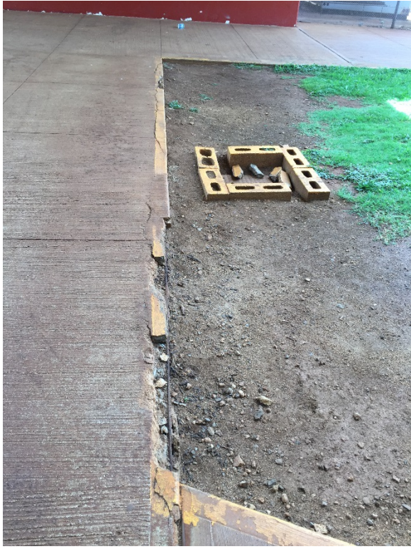
Concrete curb to be repaired
