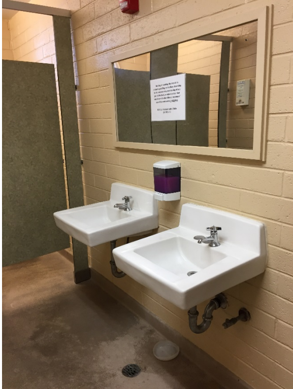
Additive alternate - replace 4 each lavatories and faucets. Note location of floor drain, Women's restroom. Contractor to ensure proper slope to the floor drain and no ponding occurs.
