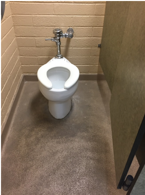
Typical restroom stall. Floor tiles only, no wall base. Concrete curb to remain. Contractor to touch up paint on concrete curb.
