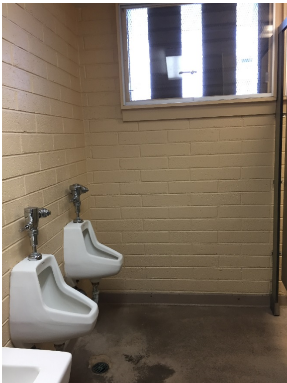
Additive alternate - replace 2 each urinals. Note location of floor drain, Men's restroom. Contractor to ensure proper slope to the floor drain and no ponding occurs.
