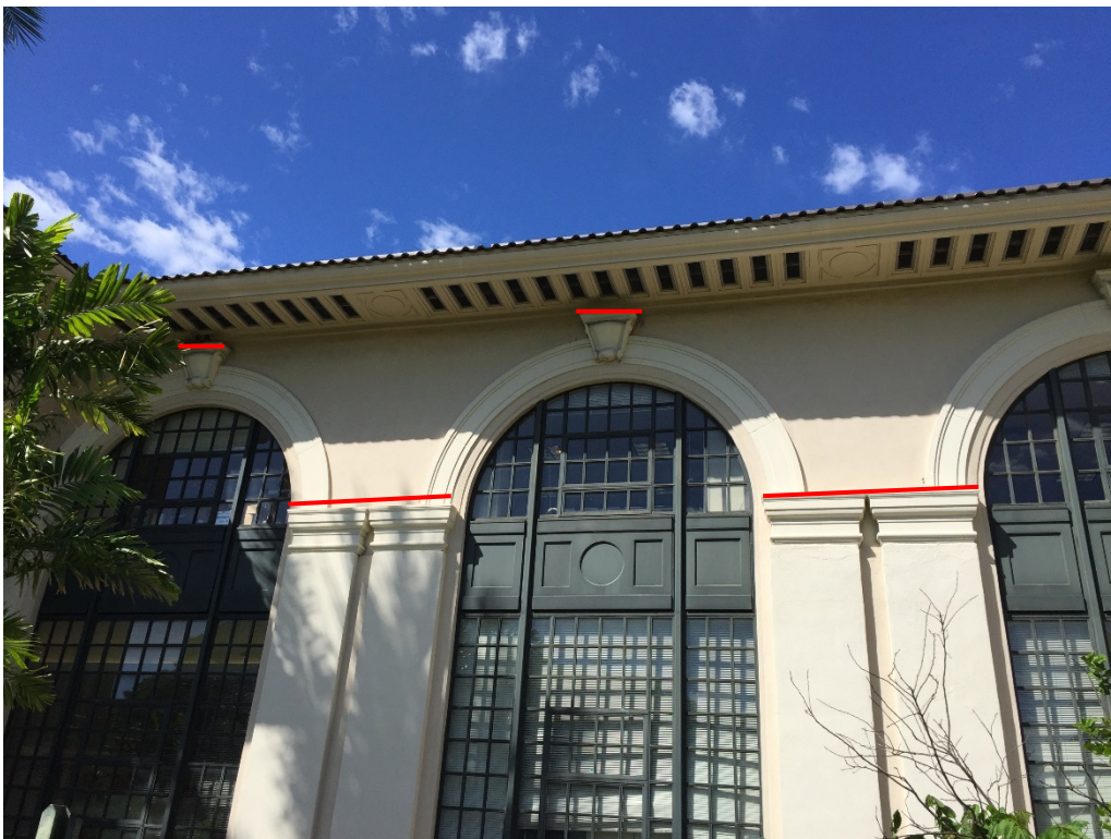
Typical voussoirs and column caps where bird spikes to be installed (outlined in red).
