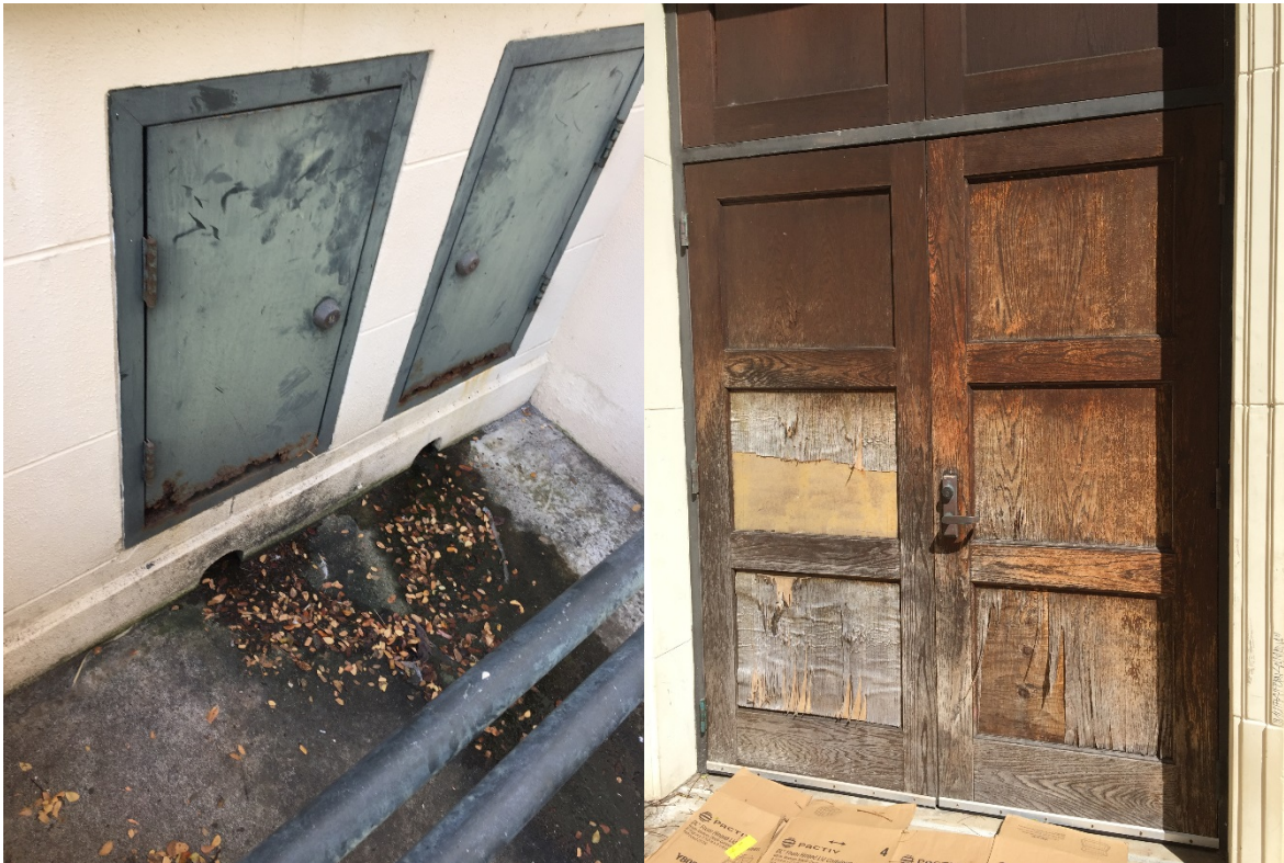
Hollow metal doors at book drop and wood door at Corridor 110 to be replaced.
