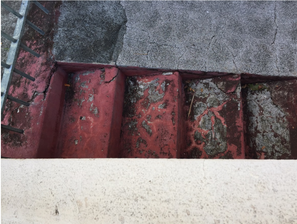
Typical minor concrete repairs necessary
