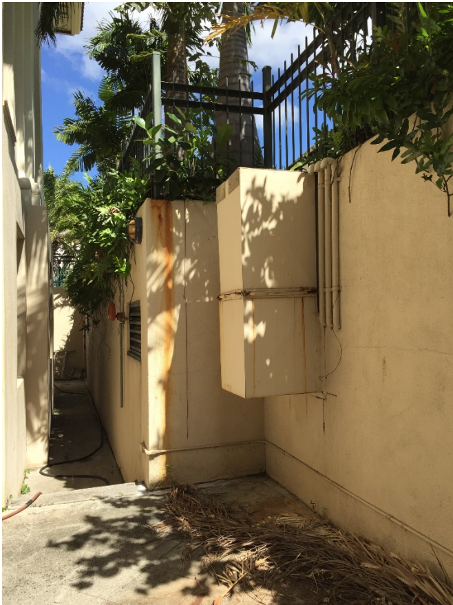
Corrosion of fence post on top of wall to be treated and painted.
