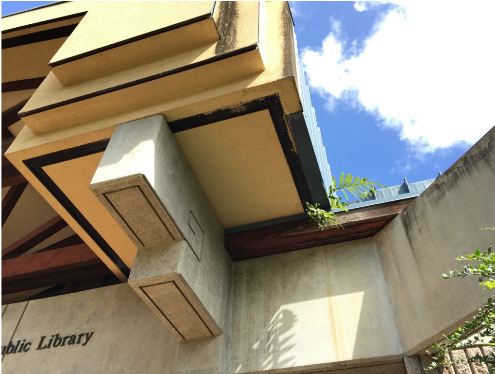
One of the wood beams requiring repair, soffit vents to be painted, moss to be removed from EFS prior to painting, and concrete beam to be cleaned.
