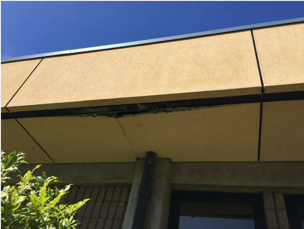
One of the soffits and vents requiring repair.
