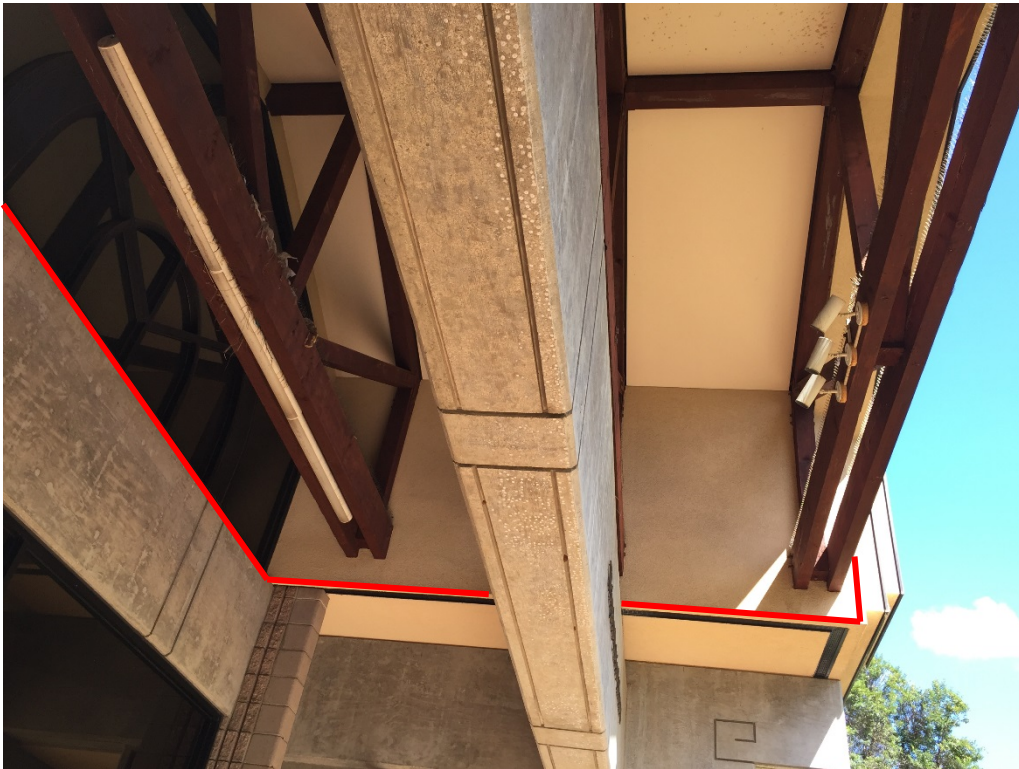
Side view of Entry area where bird netting to be installed (outlined in red).
