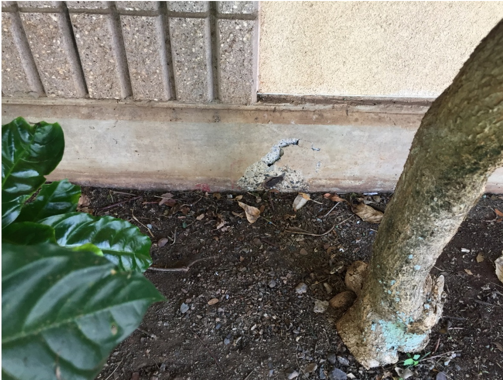
Typical, minor spall repair required
