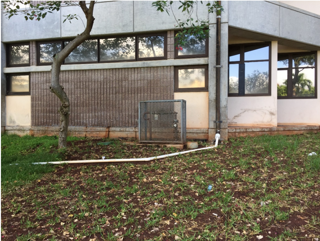
BFPA enclosure at Waipahu Civic Center. BFPA enclosures to be installed shall be of like construction.
