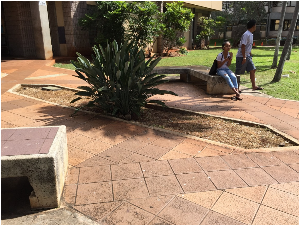
Planter area to be filled in with concrete. Utilities to the planter shall be terminated below grade. New slab to received broom finish.
