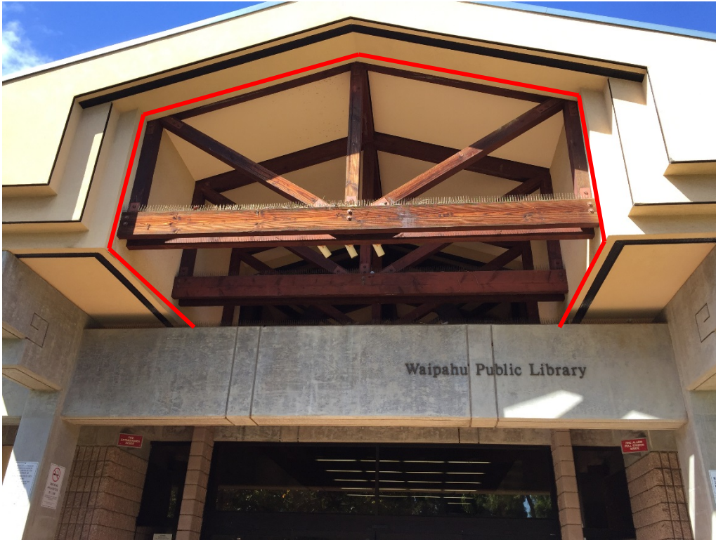
Entry area where bird netting to be installed (outlined in red). Bird spikes on top of wood beam to be removed.
