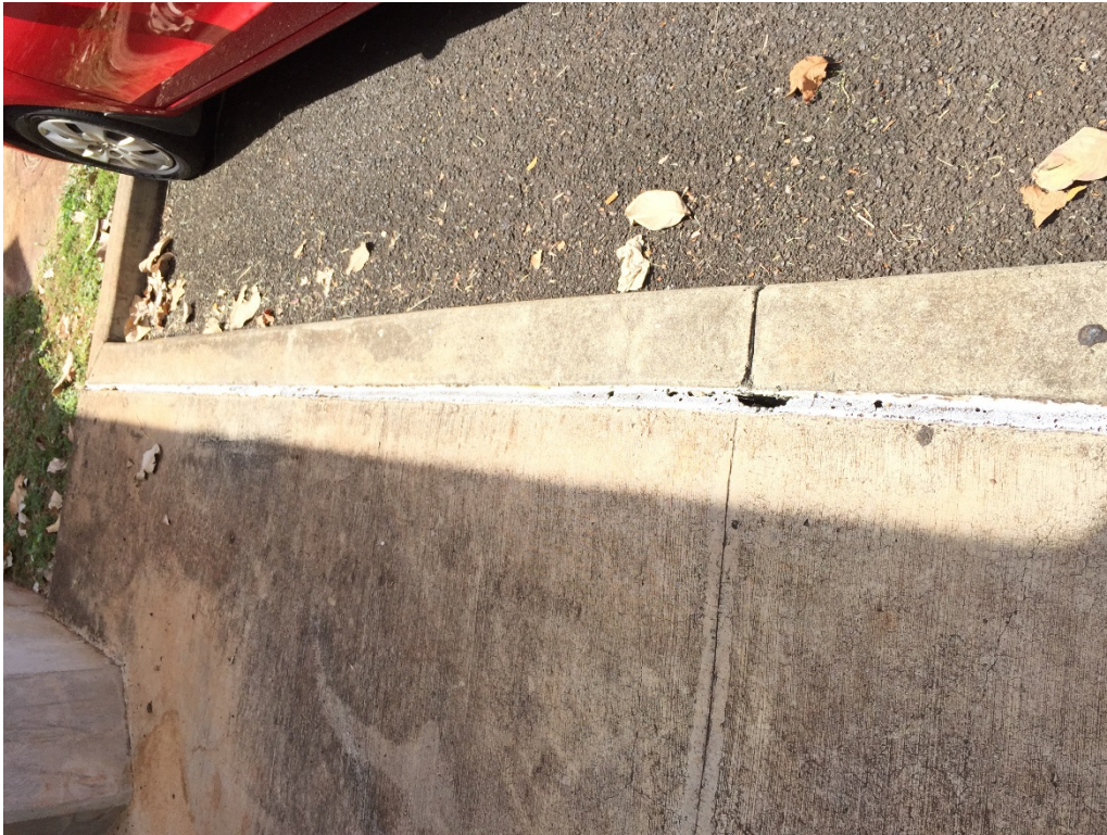
One of the control joints requiring replacement of joint sealant.
