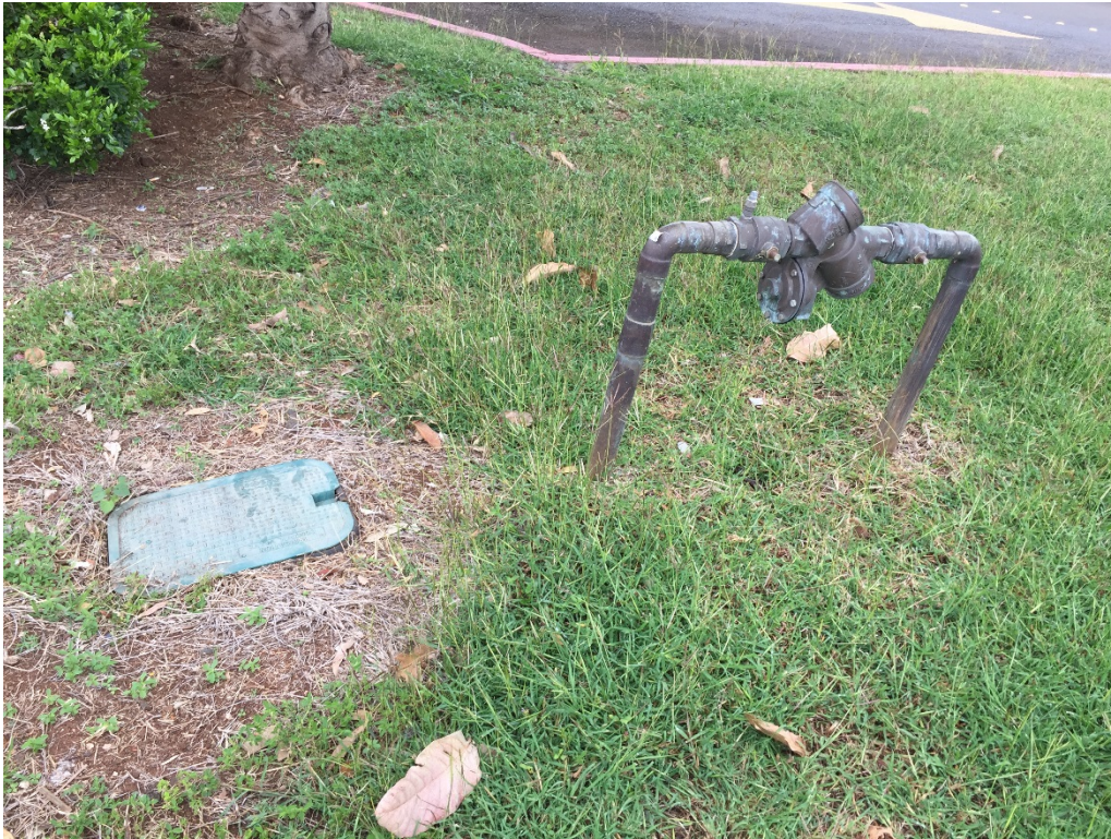
One of two BFPAs to receive enclosure. Approximate dimensions: 32"W x 27"H. Note valve box may need to be moved.
